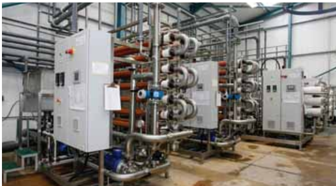
This filtration plant for Axminster Carpets, which was designed, built and commissioned by Axiom Process, is part of what is believed to be the UK's first sizeable (400m 3 /day) wastewater recycling plant (WRP) that has almost a closed loop system and target "zero discharge" to sewer.
